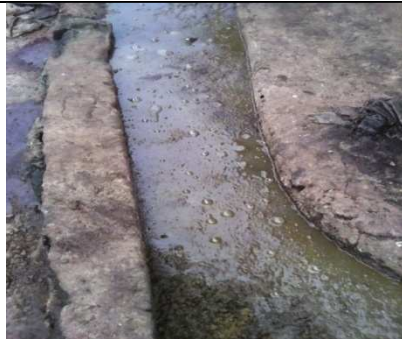
Fig 1. Stagnant gutters/ drainages
